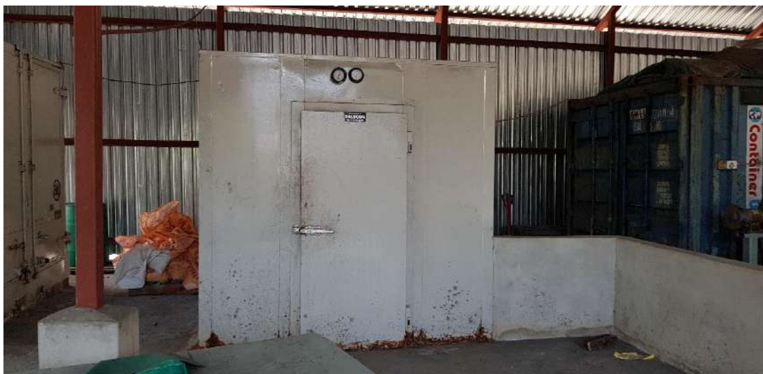
Image 8: Cold-room storage for the skins
